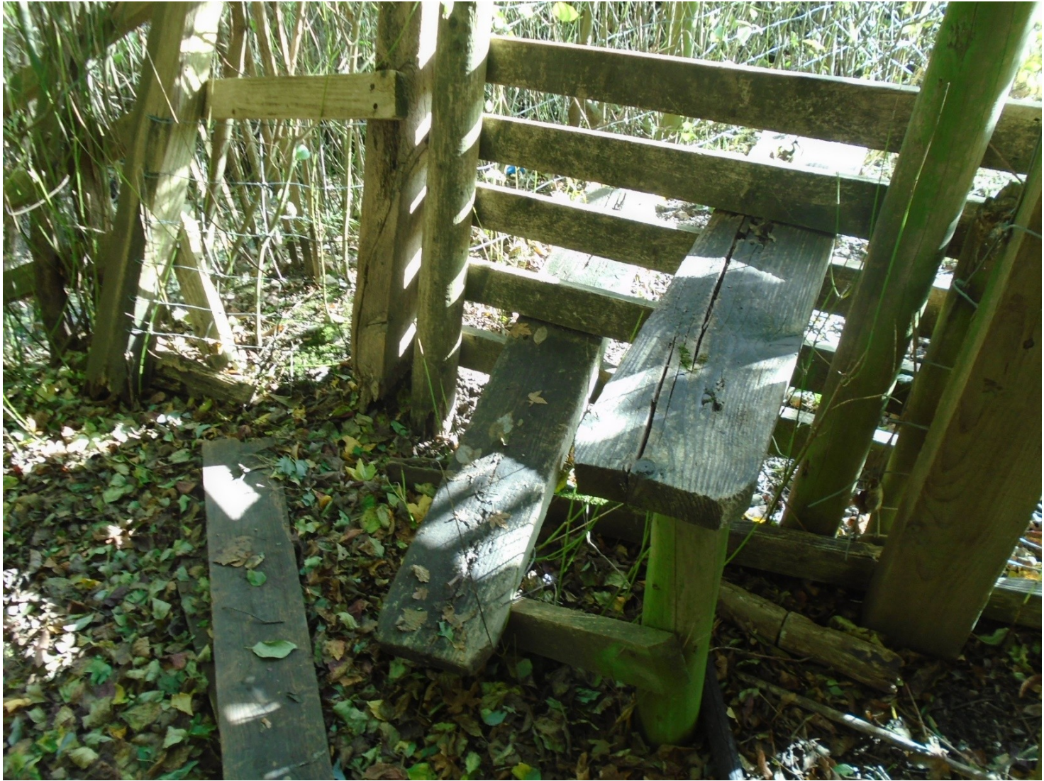
Another broken stile.
