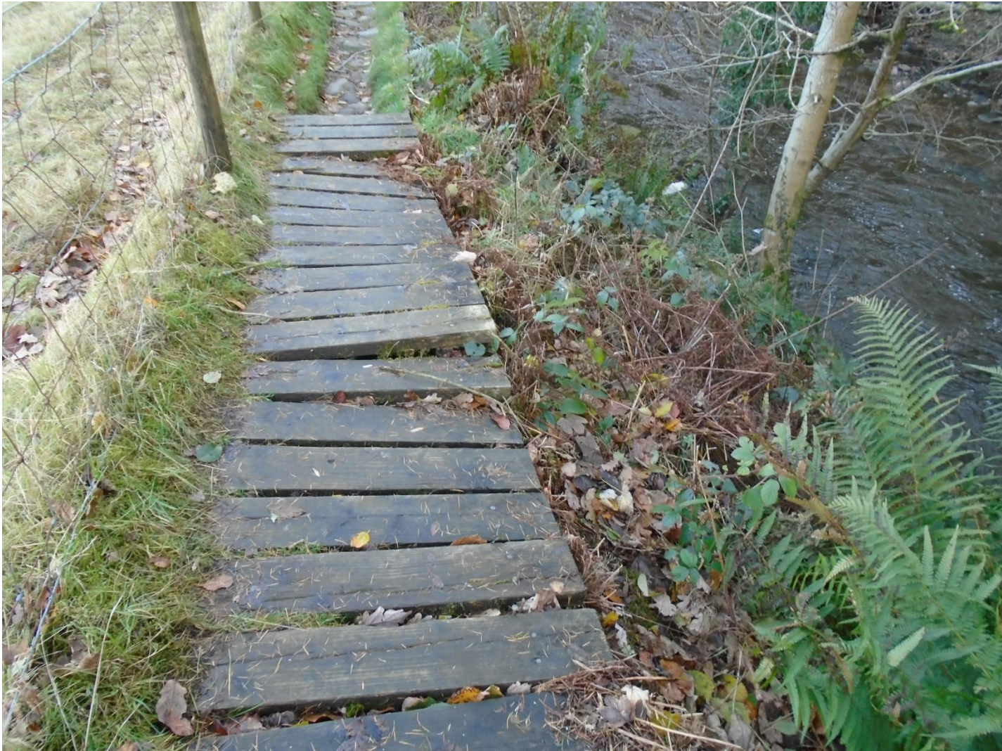
Broken board walk.
