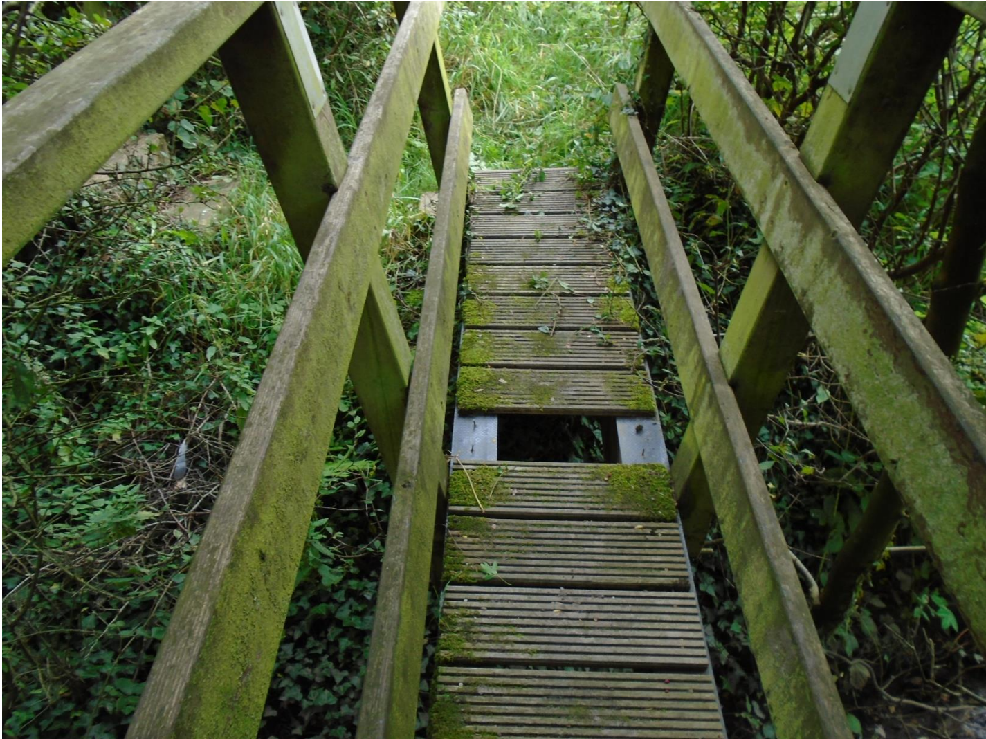
Broken decking on a footbridge.
