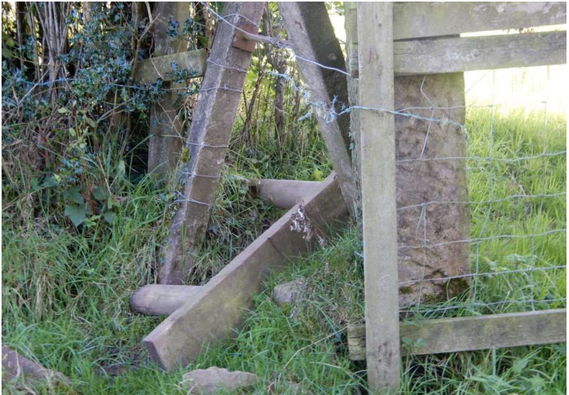
And another broken stile.
