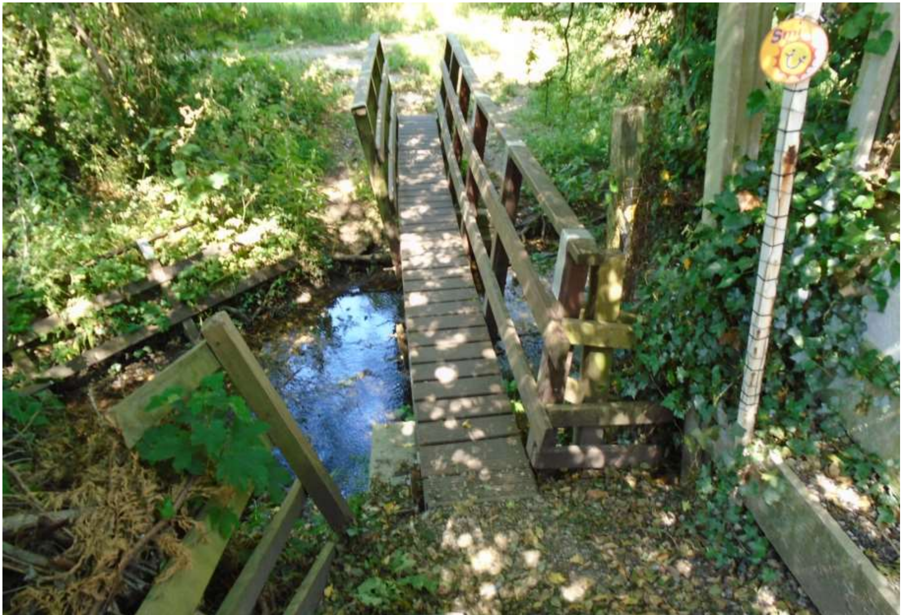
Broken rails on a footbridge.
